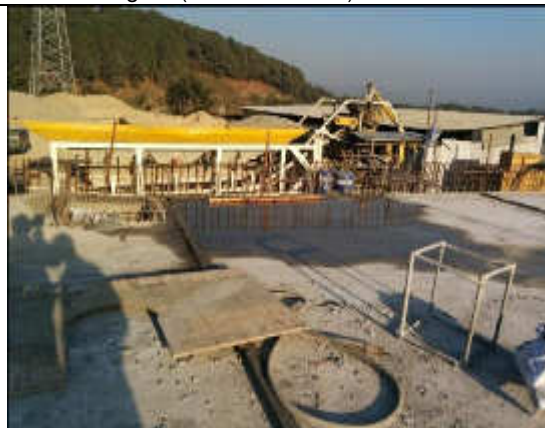
Figure 6: Batching plant at Arubari SRT, BDS Package 1
