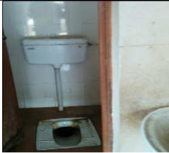
Figure 10 Toilet at Sundarighat DNI Package 3 (Sumec Lama JV)
