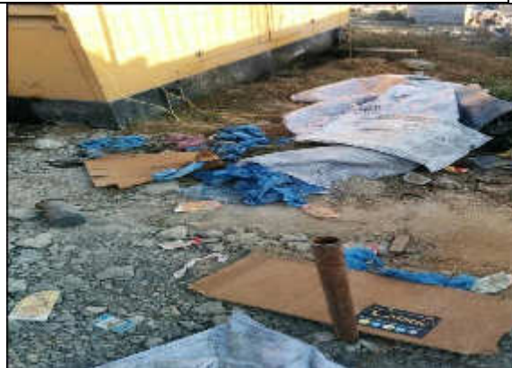
Figure 1: Cement bags not managed properly, BDS Package 2 (JWIL-SCPL JV)
