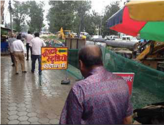
Work area is confined within barricaded area by green net, leaving space for pedestrians.
