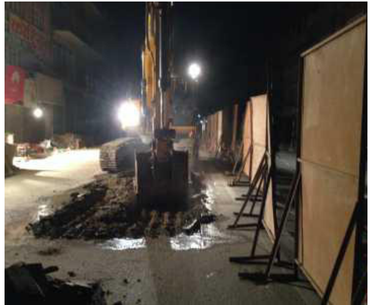
BDS-1 Bulk line Night work with Metal hoarding barricade at Chabahil on Black topped Road
